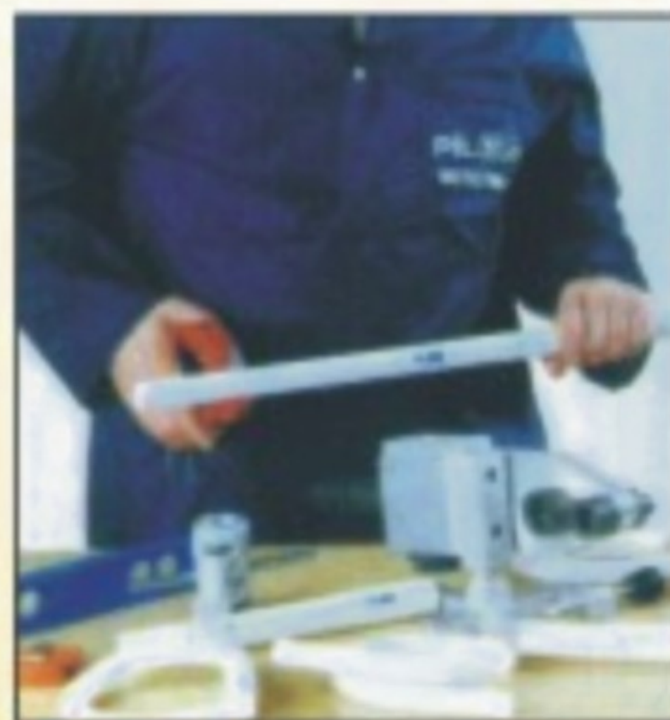
PIPES IS CUT...
